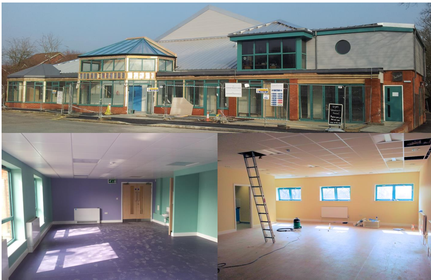
The Community Centre works are nearing completion – these photos were taken in mid-March. Clockwise from top: the front of the building, the new first-floor room and the dedicated room for the nursery
